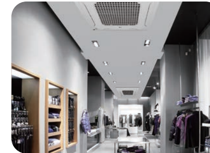
Multi-split air-conditioning systems
